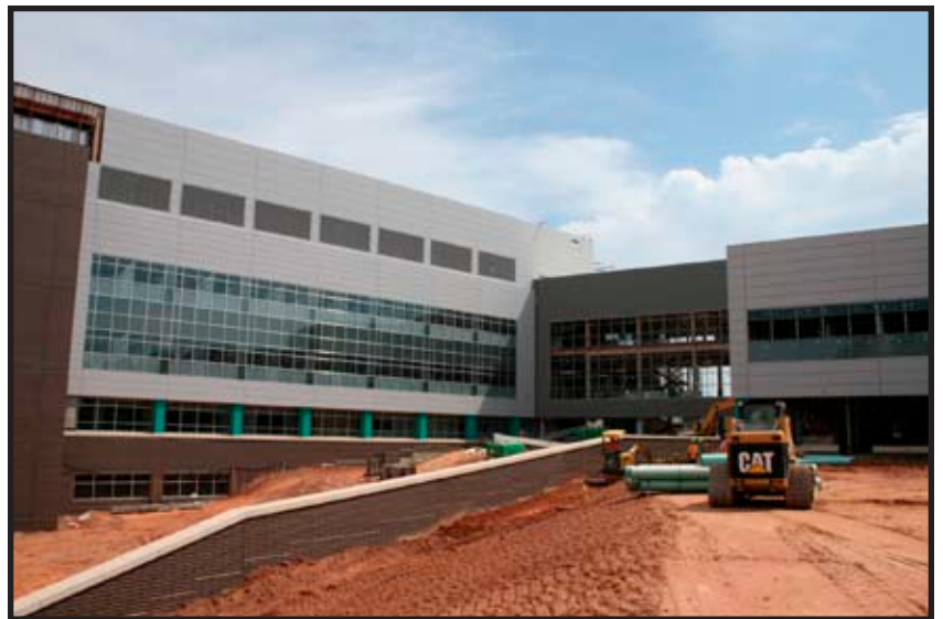
New SLPH and OCME facility, March 23, 2011, view from the back of building.
